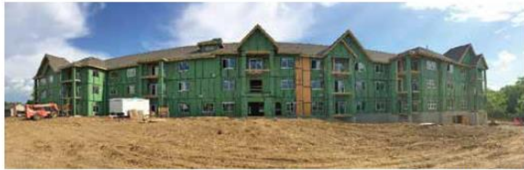
The Village Cooperative in Kansas City, Missouri, (seen here under construction) is another multifamily project preferring natural gas to electricity for heating. Each unit at the Village Cooperative has a natural gas Magic-Pak by Lennox for space heating.
