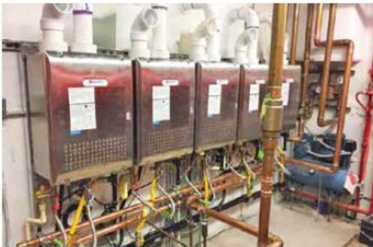
A bank of five Noritz condensing tankless water heaters are installed in a mechanical room at one end of each of the five buildings making up the 250-unit multifamily Spanos Corp. complex in Sanford, Florida. The design saves $800 per unit, or $200,000 in upfront costs.
